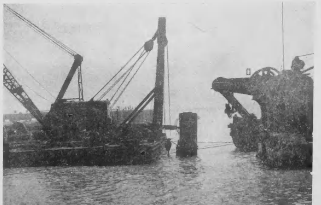
As Finger Pier No. 1 nears completion, these barges finish their work of clearing away the east end of the T dock. Here the last group of pilings is removed. It is expected that by the middle of December work will begin on Finger Pier No. 2.
